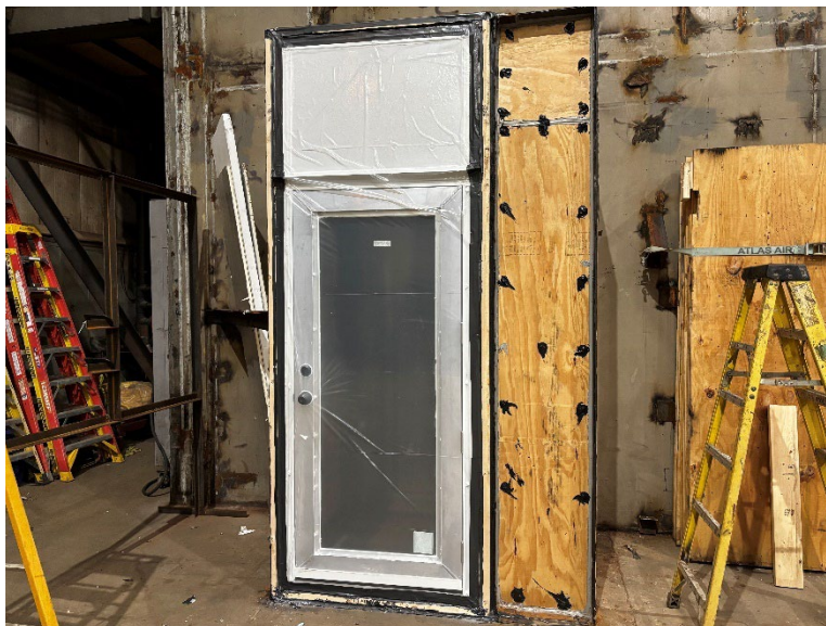
Photo No. 2 Static Air Infiltration Tare Bag
